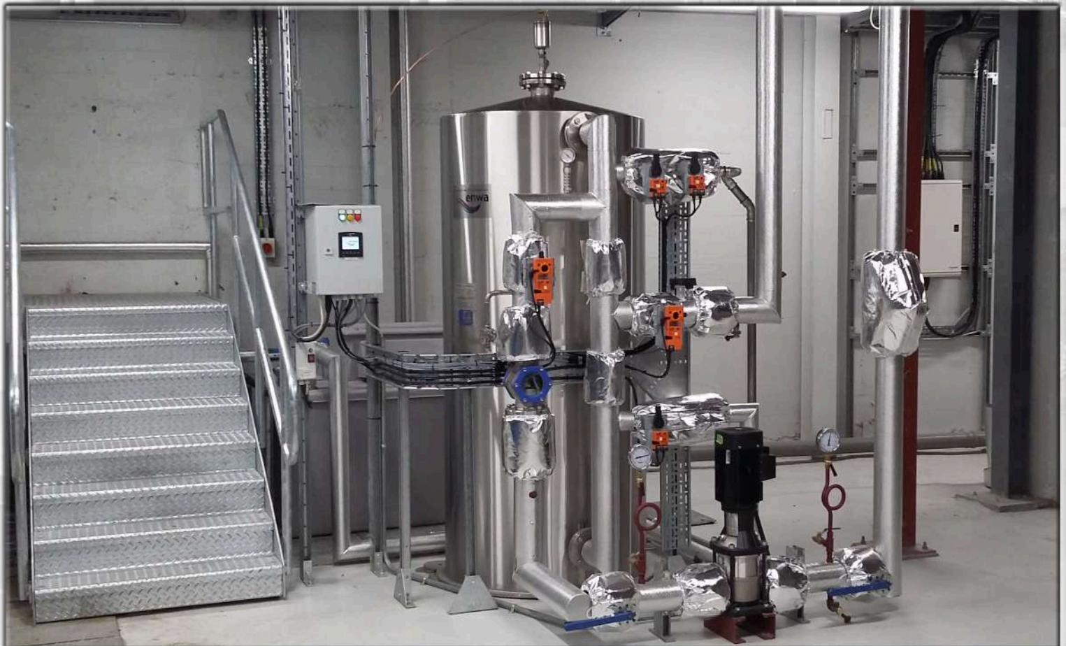
University of Glasgow - District Heating - 500 m3
